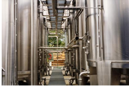
INSTALLATION CUVERIE - REUNION
