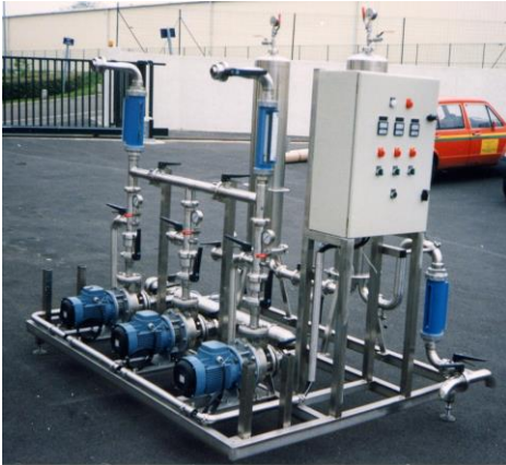
STATION DE POMPAGE TAHITI
